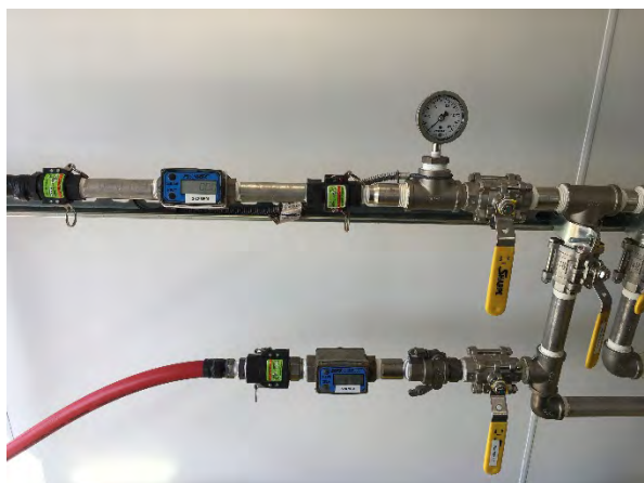
Injection Flow and Pressure Monitoring
