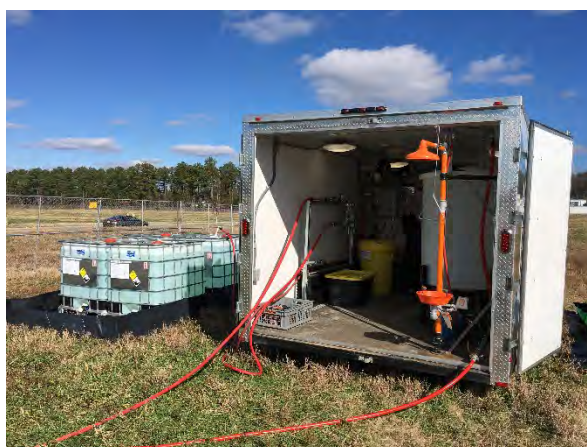
Injection System / Safety Shower & Eye Wash
